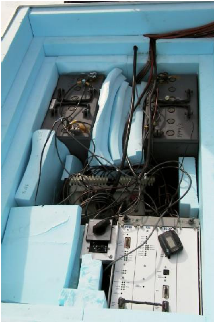
Figure 4: The GPS instrument box in 2000-2001, showing how the insulation material has begun to melt. (Photo Eija Kärkäs)
